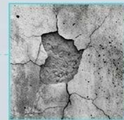
Medium Spalling + Noise
